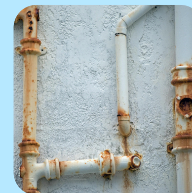
Old facilities, rusty pipes
